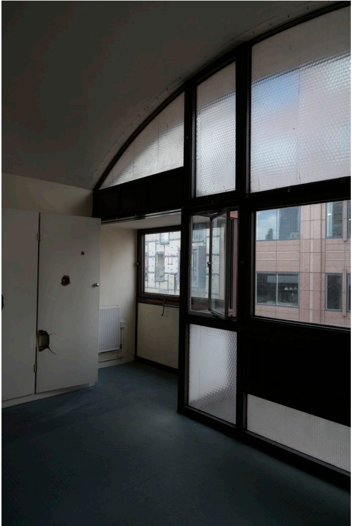
Image 9 – internal view of Flat 347 Oriel window
