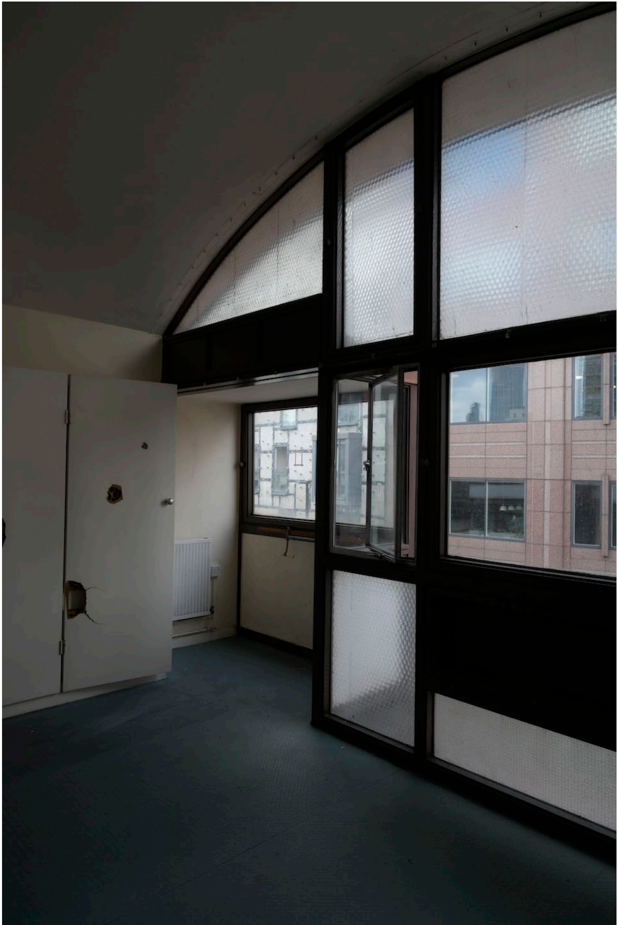
Image 9 – internal view of Flat 347 Oriel window
